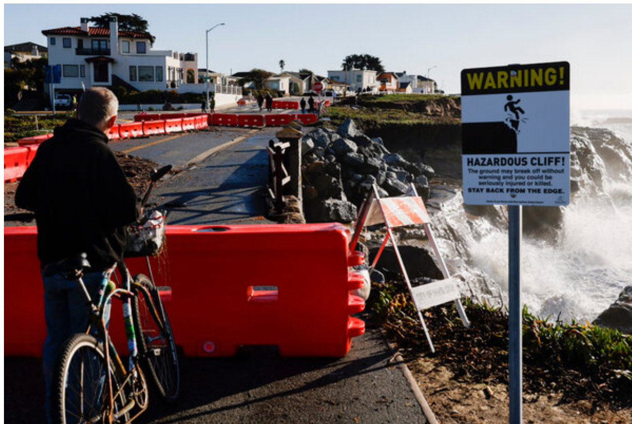
Barricades blocking off a crumbling section of West Cliff Drive in Santa Cruz in January. Jessica Christian/San Francisco Chronicle, via Associated Press
